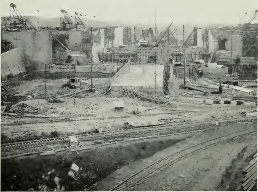
ABOVE, SPILLWAY AND FOUNDATION OF GATUN LOCKS. LOWER PICTURE, LOOKING NORTH IN GATUN LOCKS.
